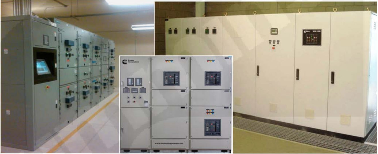
FIGURE 23. EXAMPLES OF SWITCHBOARD/SWITCHGEAR EQUIPMENT IN NORTH AMERICAN, SOUTH AMERICAN, AND IEC-BASED DESIGNS.
