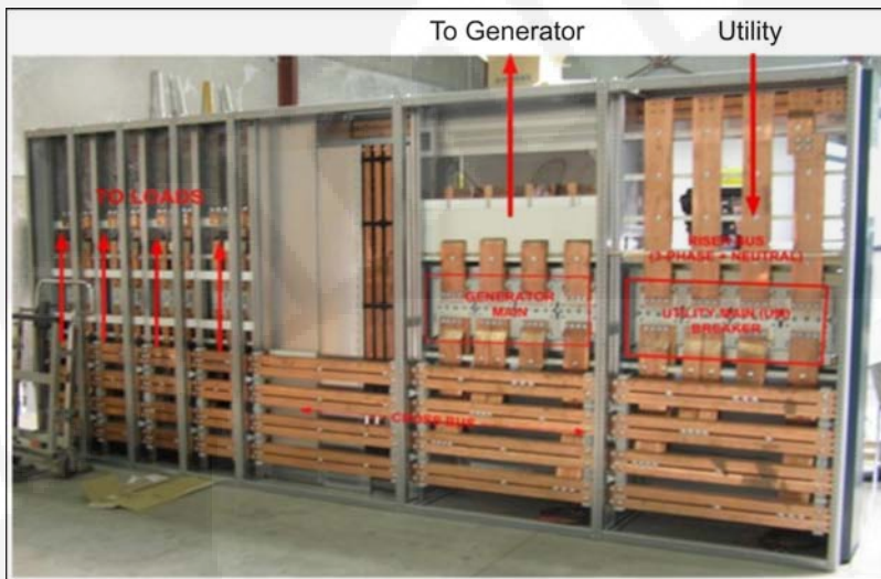
FIGURE 30. VERTICAL BUS STRUCTURE (CROSS BUS BARS ABOVE EACH OTHER) IN AN IEC SWITCHBOARD DESIGN
