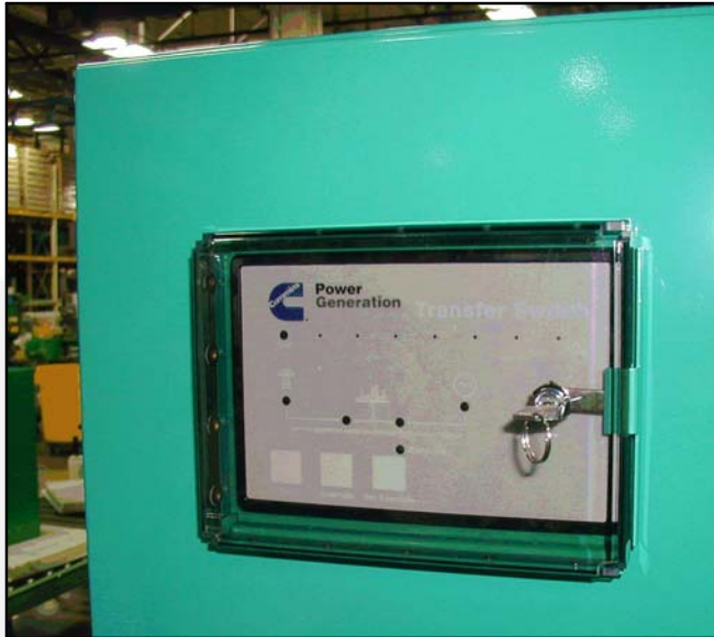
FIGURE 3-20. INSTALLED CONTROL PANEL COVER GUARD
